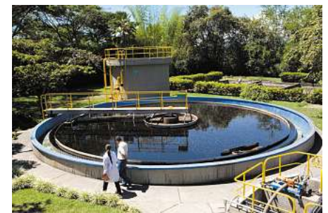
The wastewater treatment plant at our Bugalagrande factory in Colombia, one of our 292 facilities worldwide.
