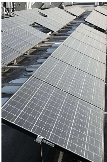
In addition to improving energy efficiency at its Denver factory, Nestlé Purina PetCare now generates 1% of its electricity needs from solar power.
